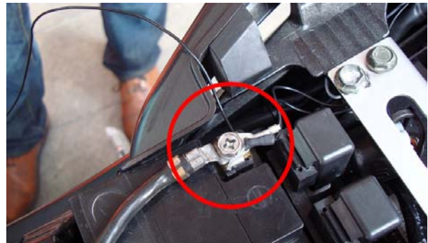
Figure 17: external ground cable is correctly connected.
